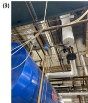
Boiler Room Trap #83 Created: Tue, 4/30/2024 Installed incorrectly, failed open.
