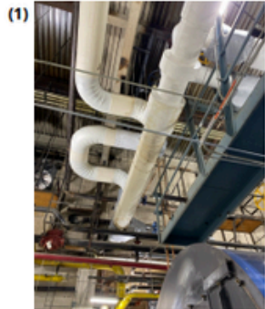
Boiler Room Header For Main Steam Created: Tue, 4/30/2024 No Drip Traps At All On Main Header
